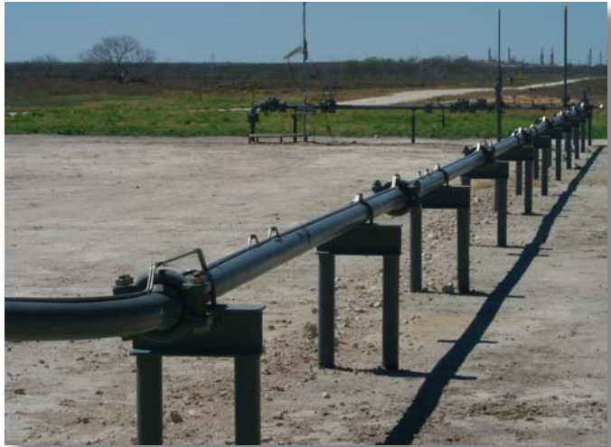
3.1/16" API 15000 psi Flowline
