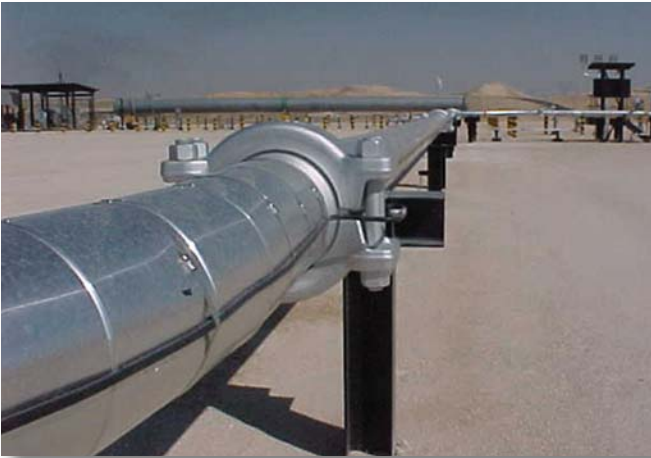
API 10000 psi Flowline
