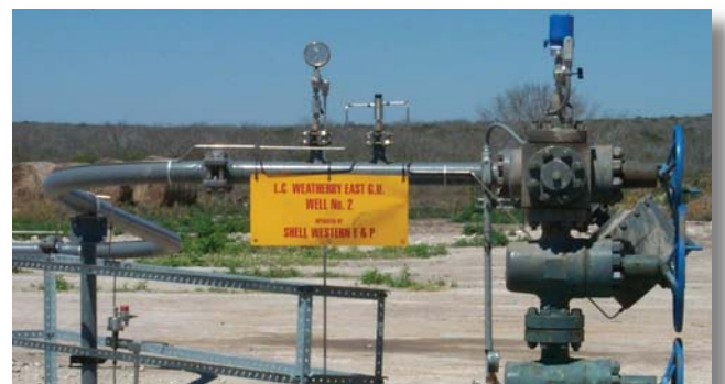
15000 psi Corrosion & Injector Assemblies
